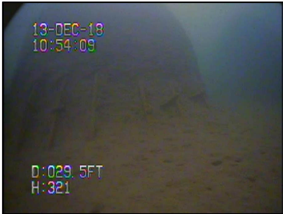
Figure 11 Erosion and rebar found on the downstream side of baffle blocks.
